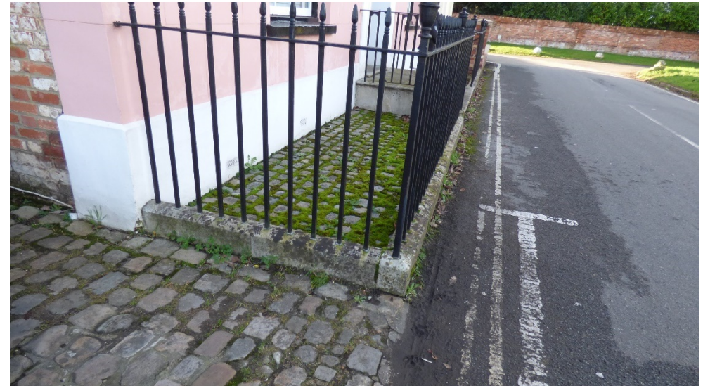
Figure 20: The sandstone paving setts outside Englewick are the only examples of historic paving in the Conservation Area.
